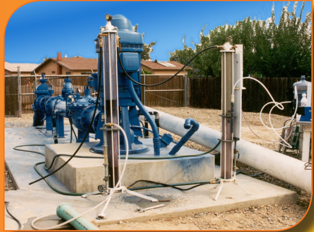
3" Iron & Manganese well water pilot test
